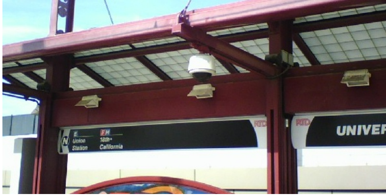
Figure 3: Dome-Enclosed Surveillance Camera at the University of Denver Light Rail Station 85
