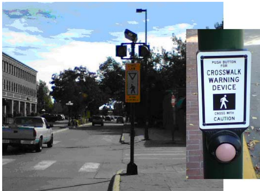
Figure 1: Recent Photograph of Solar Powered Crosswalk Warning Device and Button on Main Street in Parker, Colorado 60
